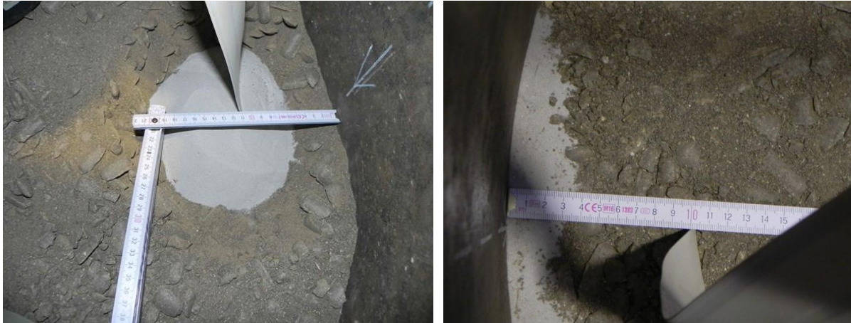
Figure 4.48 HTV-6 – sand lenses for the simulation of local fault zone in bentonite (left) and artificial EDZ with sand (right)
