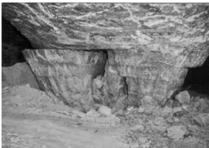
Figure 2. Softening phenomena within the rock and on horizontal bedding planes of a hard salt pillar.
